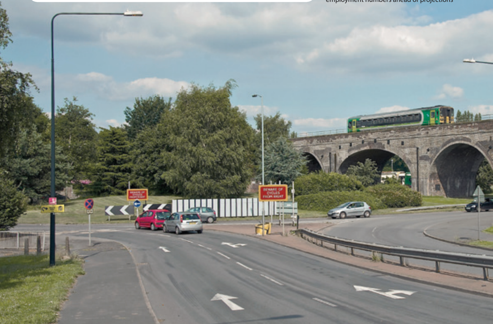
Coton arches: the one major engineering structure on the Coventry to Nuneaton line has recently been repointed. Unit No 153366 crosses the arches on 21 July 2014. John Whitehouse
